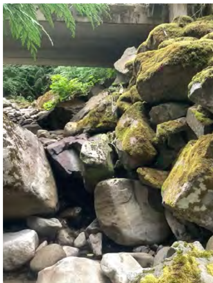
Riprap and scour left bank
